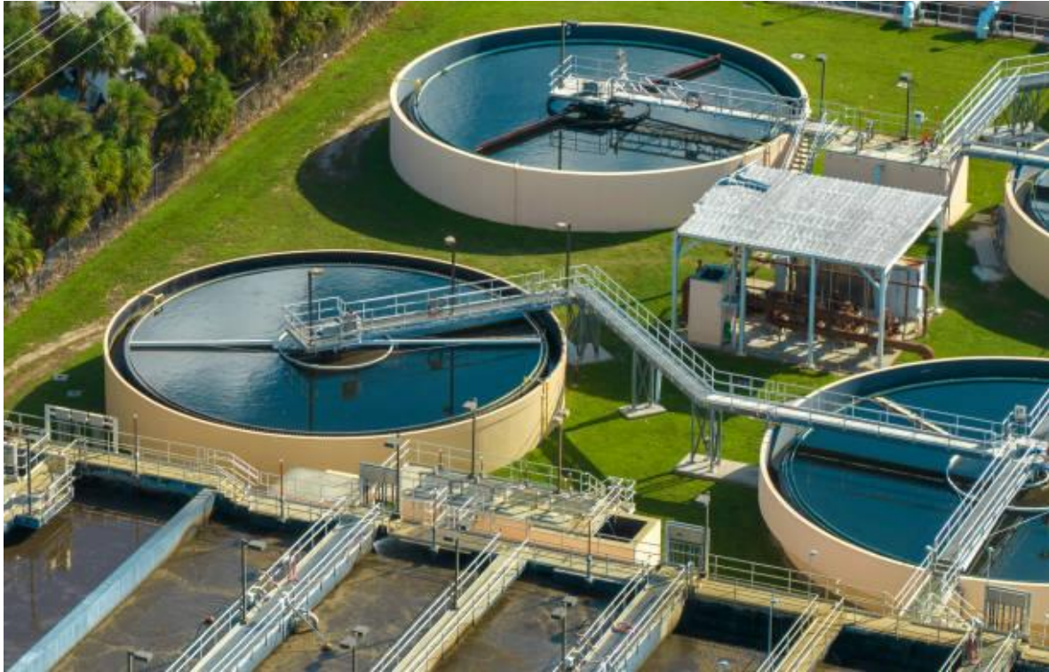
Figure 1.7 – Water treatment plant
