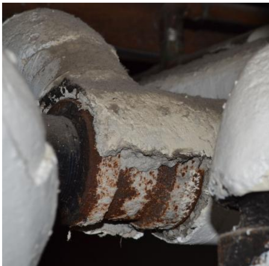
Figure 6.4. The figure shows a damaged asbestos pipe wrap. While this use of asbestos is banned in the United States, other uses are still permitted. Image by EPA (public domain); Supplemental reading: Learn About Asbestos | US EPA .
