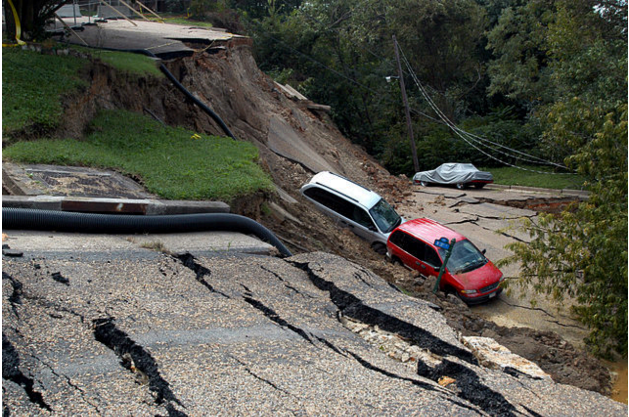
Figure 6.7. This figure shows the section of E. Grace Street, Richmond, VA, collapsed during tropical storm Gaston. Gaston dropped twelve inches of rain in the area. Image by Liz Roll/FEMA Photo Library (public domain).
