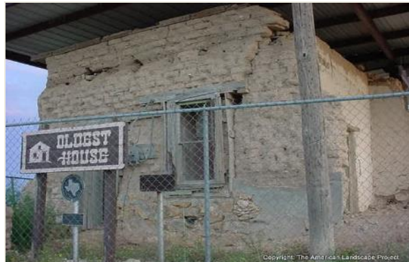
Figure 2-30: Fort Stockton, TX - This house built in the mid-19th century has fallen on hard times. Adobe bricks deteriorate when exposed to rain.
