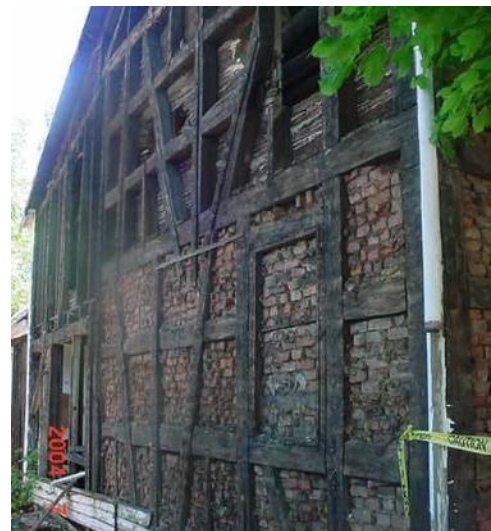
Figure 2-4: Chillicothe, OH. This house was built using hand-hewn heavy timbers with brick infill. This method of construction is replaced by the mid-1800s in the US by new, popular techniques.
