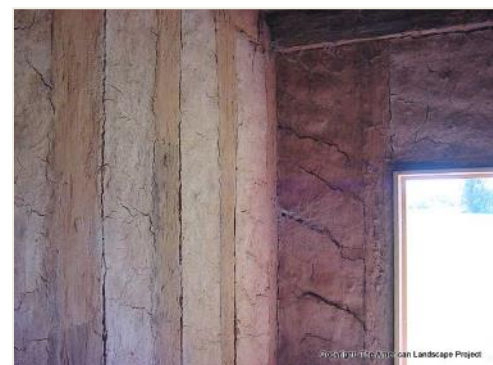
Figure 2-22: Natchez, LA - Restoration of this creole cottage revealed vertical timbers filled with bousillage.
