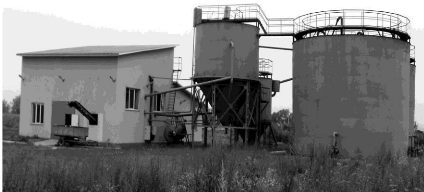
General view of the treatment facilities of the enterprise for the production of concentrated apple juice
