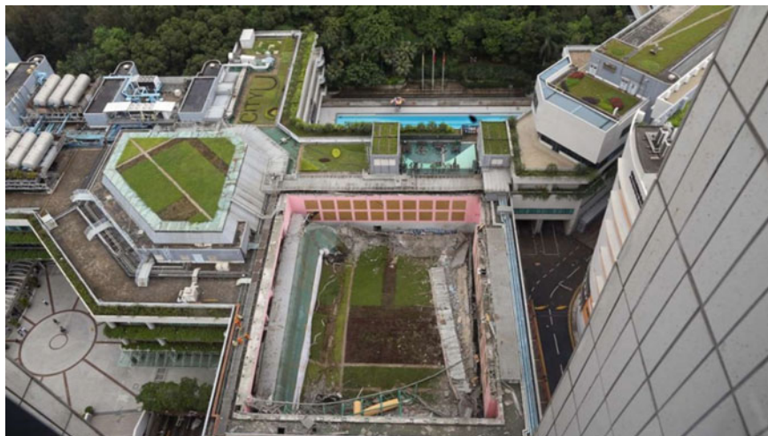
Fig. 3 The collapse of green roof at Hong Kong City University (Yau et al. 2016)
